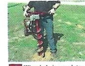
8 When hole is complete stop auger and pull out for clean hole.
